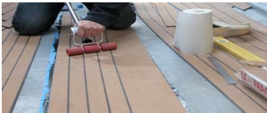
Four lengths of WDK100 joined together with Stelmax and laid in one operation. Once in place this is rolled to ensure no air bubbles and good seating on to the adhesive.
